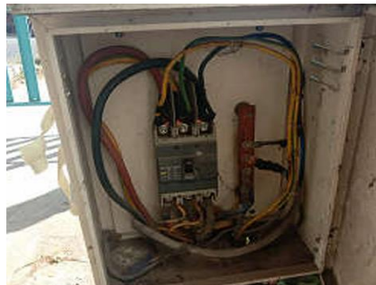
Gambar 4. Kondisi Panel MDP.
