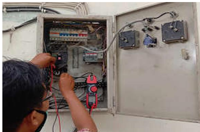
Gambar 5. Kondisi Panel SDP.
