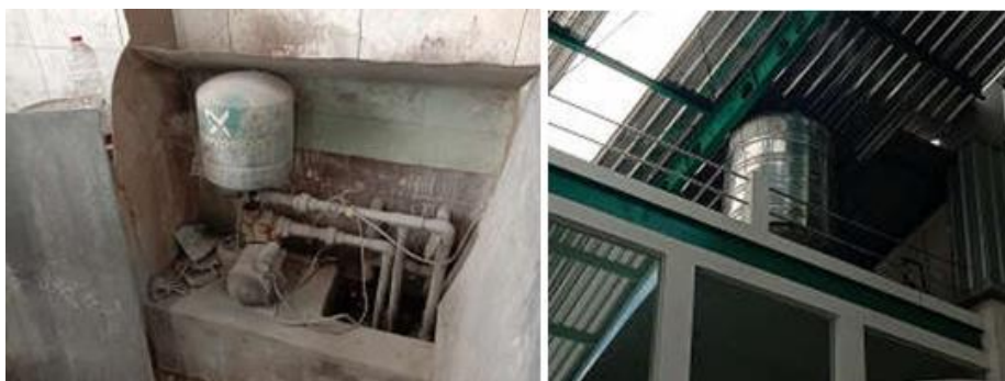
Gambar 8. Kondisi Instalasi Plumbing.
