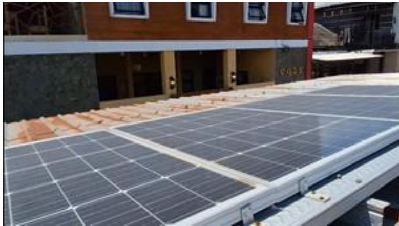
Gambar 3. Solar Panel Terpasang.
